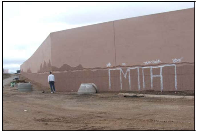
Sound walls under construction along I-80 near Oddie Boulevard in Reno. This newly built wall has become a target for graffiti.
